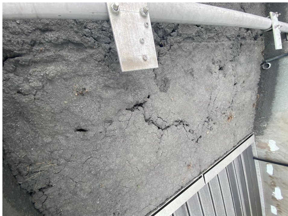
Figure 4.18: Photographs illustrating (A) the unsaturated and desiccated nature of the lower slope region one hour post-E1 and (B) the closure of secondary cracks and increased surface saturation in the lower slope after gravitational moisture redistribution and assistance from a small natural rainfall event.
