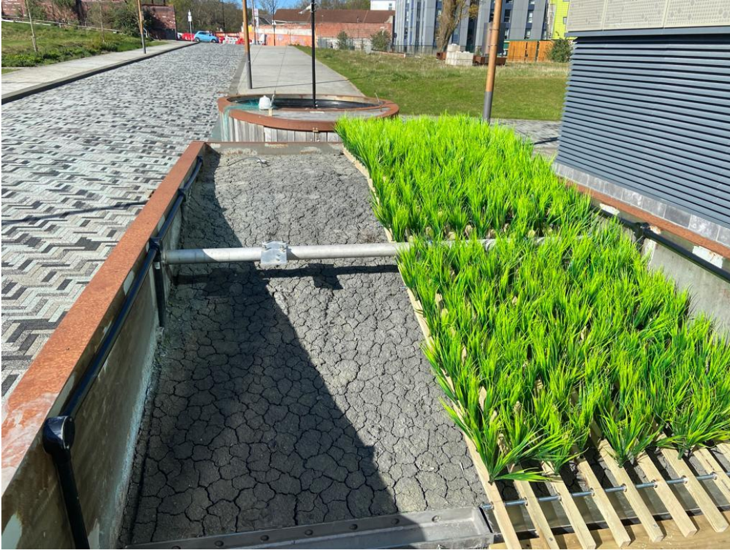
Figure 3.17: Photograph illustrating the final installation of the faux grass canopy over Side B of the lysimeter slope on April 20th 2023.
