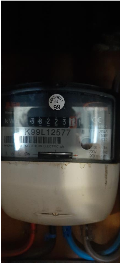
Figure 27: An electric meter.
