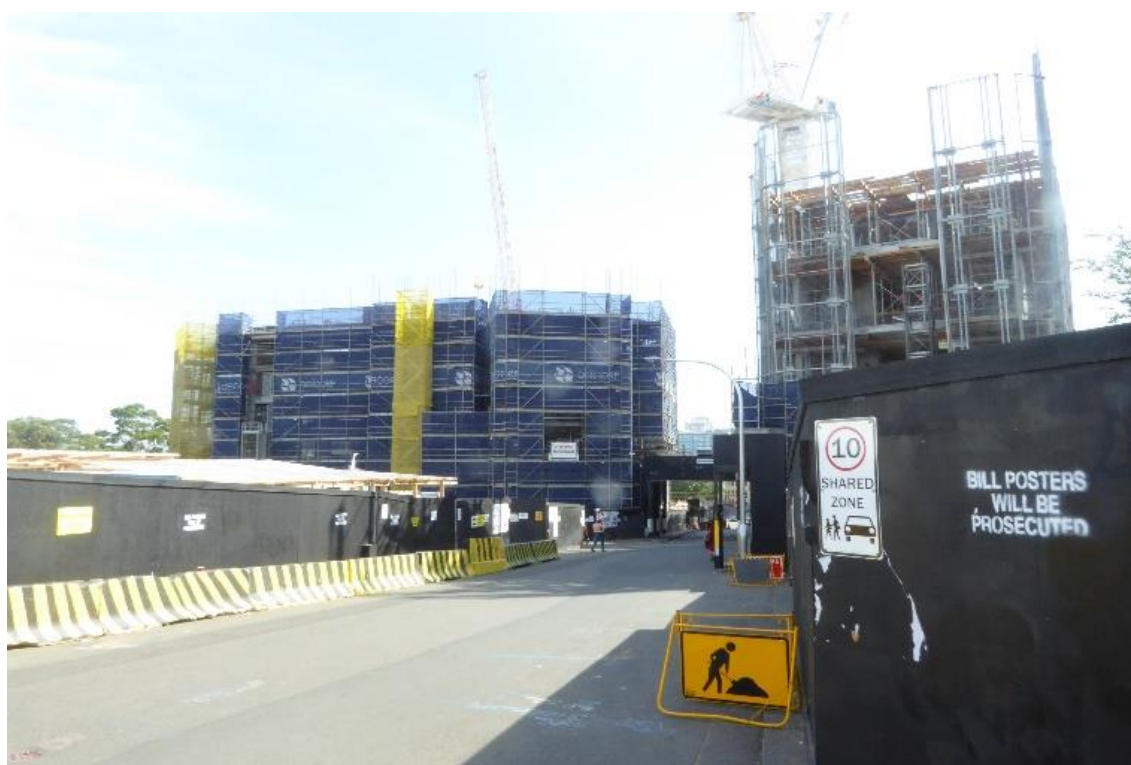
Figure 13 Student accommodation building work taking place at the site where The Block once stood
