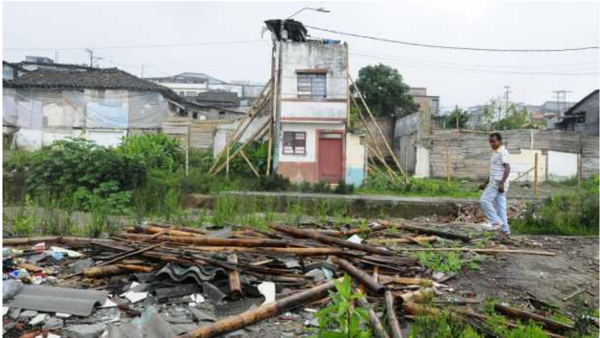
Image 16 Structures at risk in San Jose. (source: participants' archive)
