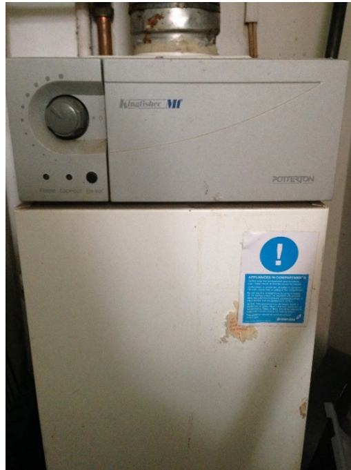
Figure 4.45 The old floor mounted fan assisted gas boiler in the Conventional House.
