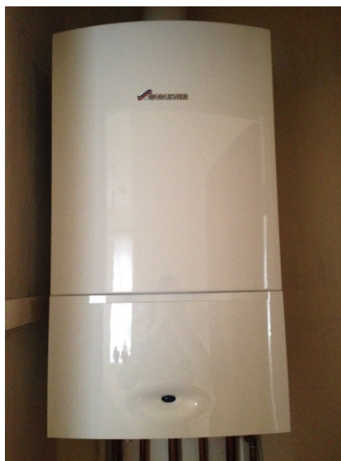
Figure 6.4 The new condensing gas boiler installed in the Conventional House.
