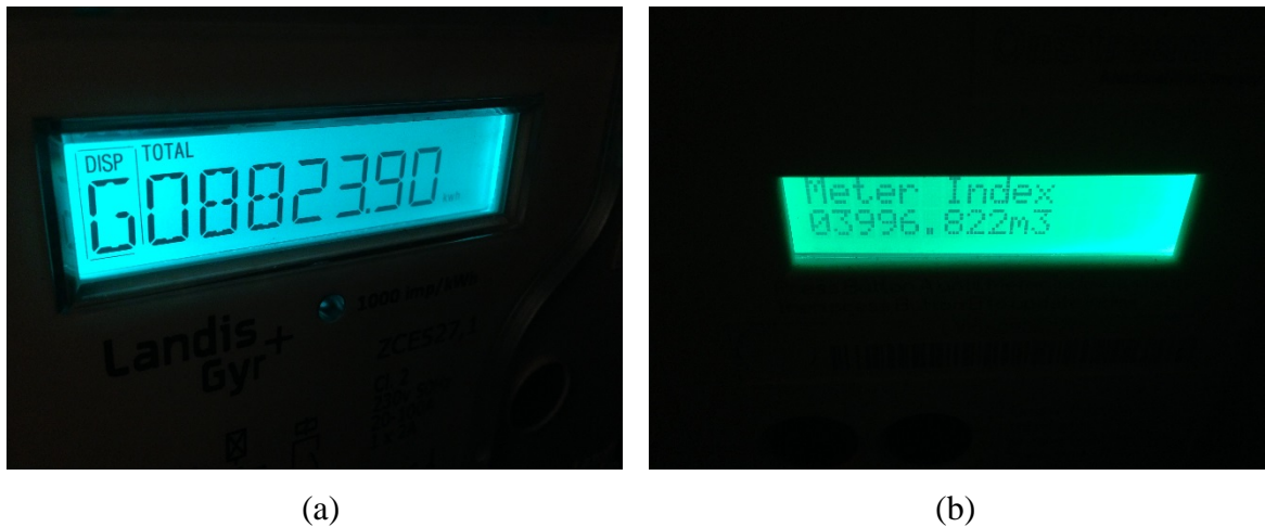
Figure 4.7 Meter readings recording during pre-monitoring period: (a) Electricity meter, (b) Gas meter.
