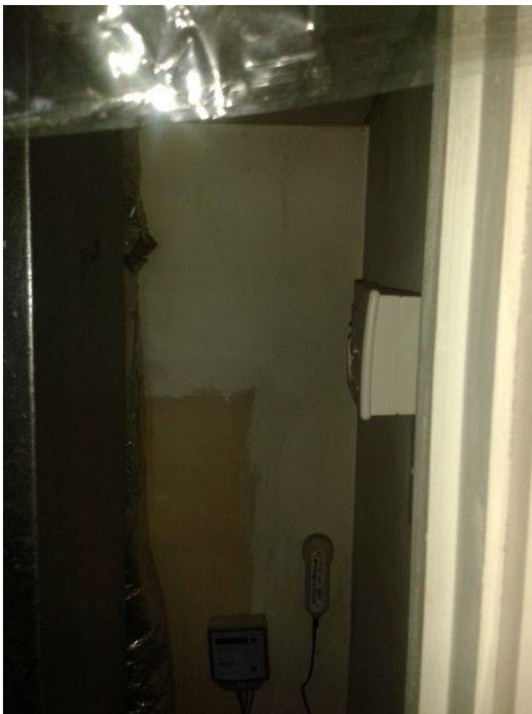
Figure Annex D. Heating controls in the target building
