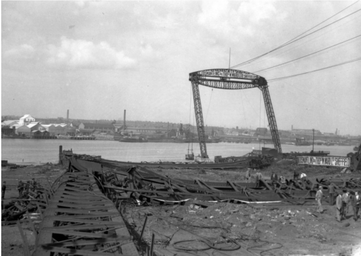
Photo 4.3: Palmers Shipbuilding's shipyard in Jarrow, dismantled by Thomas W Ward Ltd of Sheffield 203
