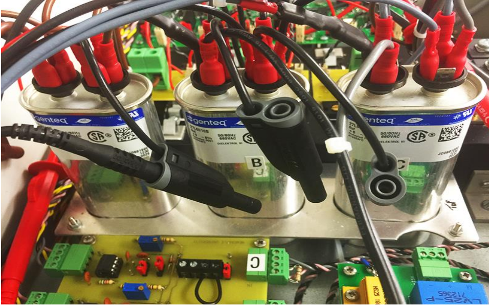
Figure E.3 Photograph of AC capacitor
