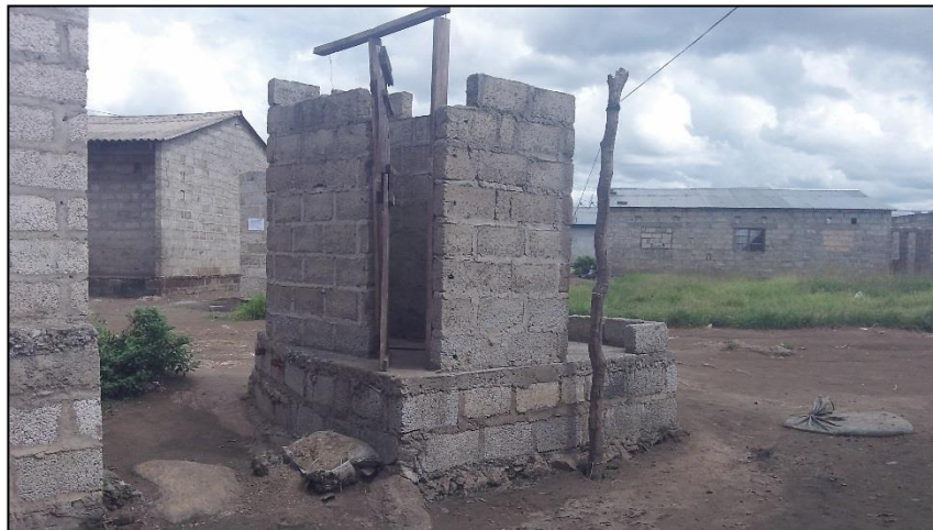
Figure 10-2: Typical pit latrine design- picture taken in Kanyama
