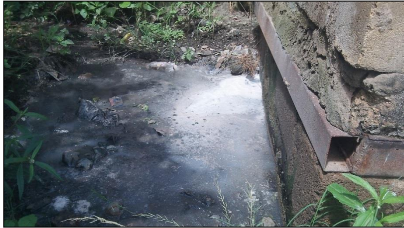
Figure 10-6: Pooling of water adjacent to a pit latrine observed in George
