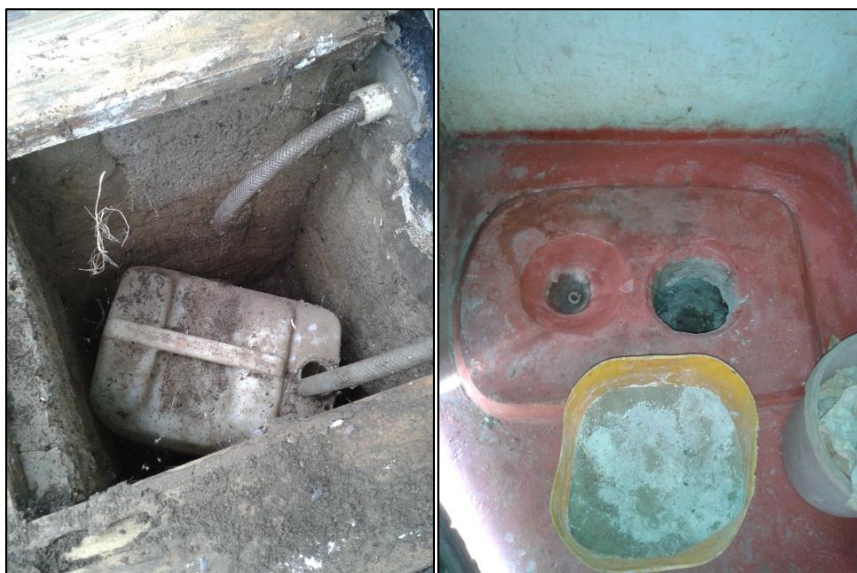
Figure 4-8: Ecosan (dry) toilet in informal settlement of George Urine collection (left), urine diverting slab (right) 3
