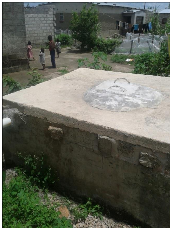
Figure 10-7: Typical septic tank design observed- picture taken in Kanyama
