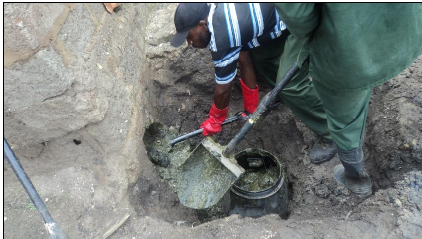
Figure 10-1: Formalised Pit Emptying Service in Kanyama
