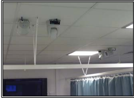
Figure 58: The fixed mounted, fully maneuverable high definition cameras installed in the SMOTS examining bays
