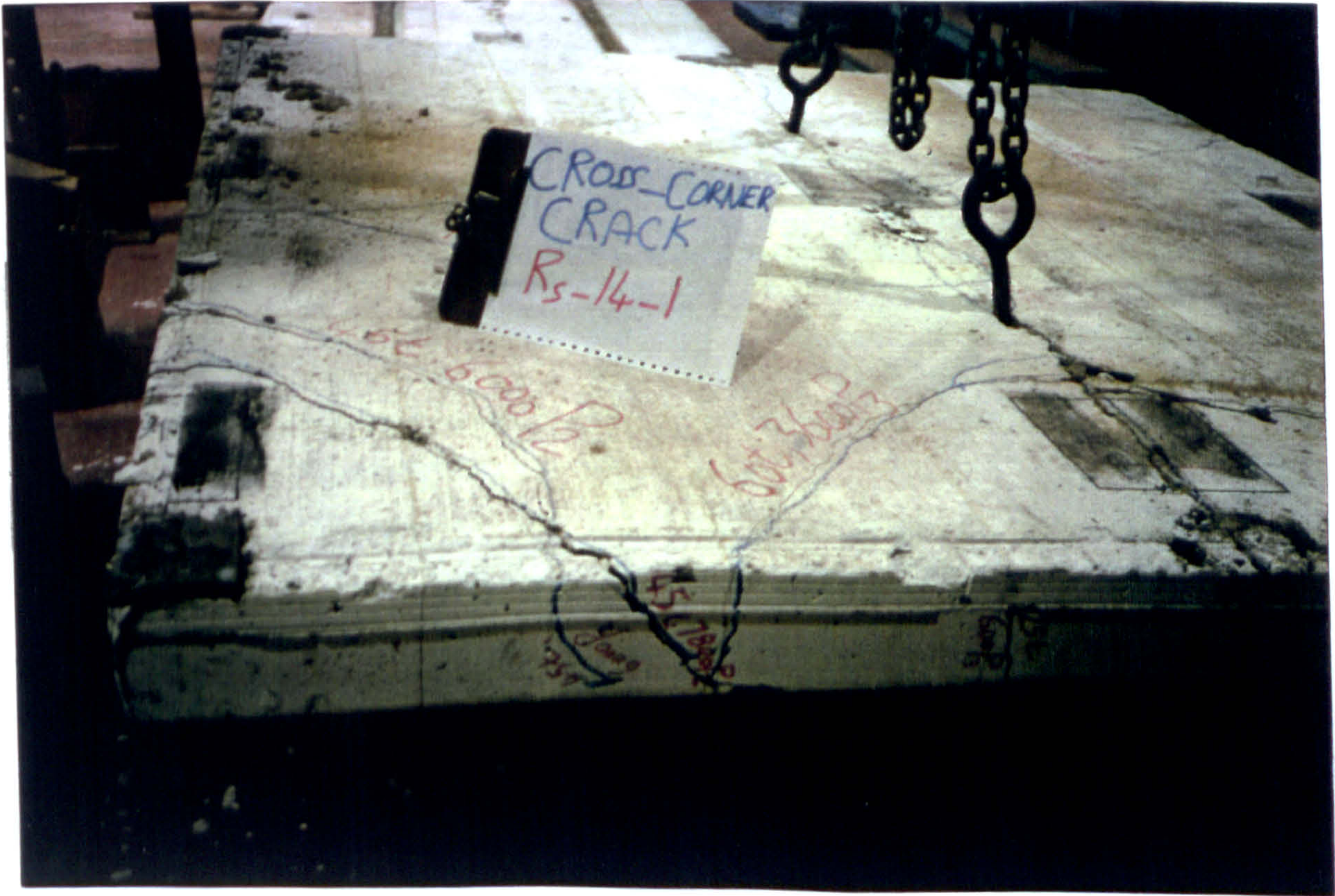
PLATE 7.3 : Combination of Punching Shear and Fatigue Fracture Failure at P3 of Raft RS1 - Module M3
