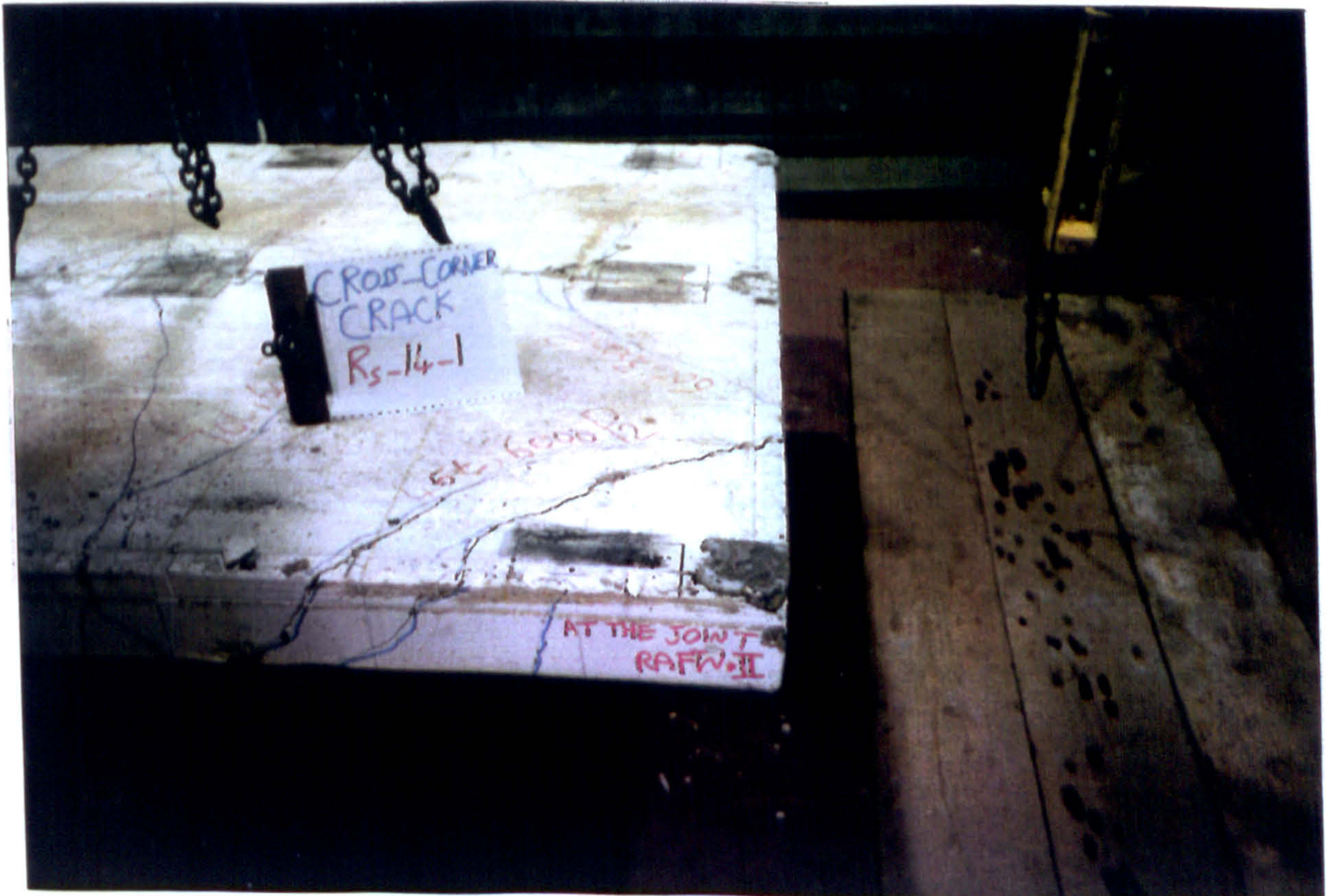
PLATE 7.4 : Cross Corner Crack at the Joint Interface
