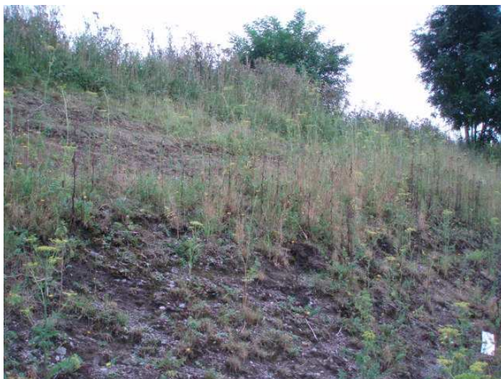
Photo 5.3. A38. South-facing bareground, signs of surface erosion.
