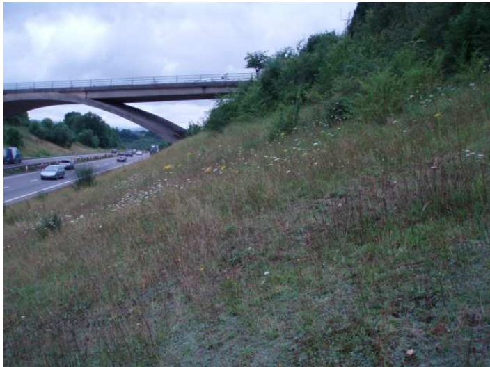
Photo 5.5. A303. South-facing bareground, signs of surface erosion.
