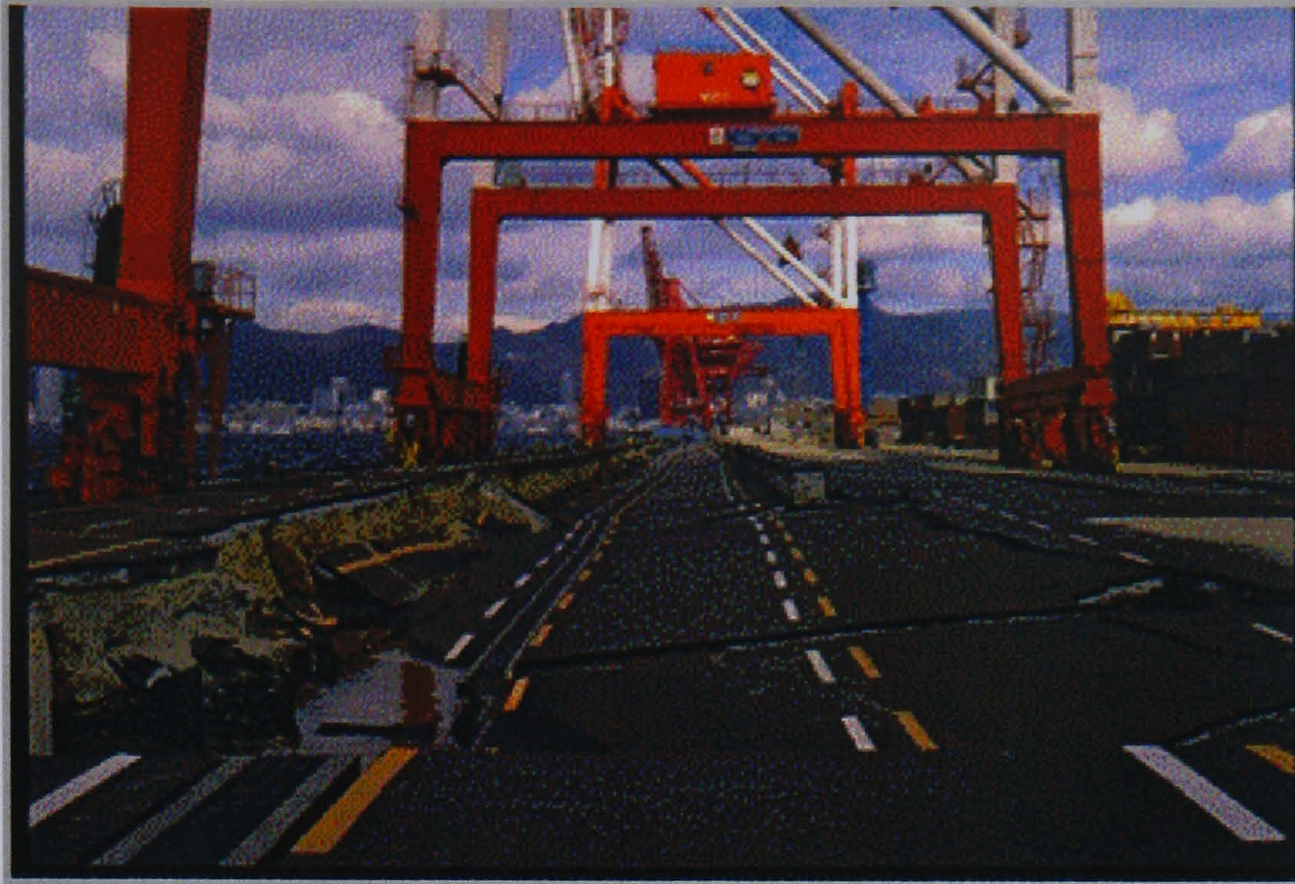
Figure 1.1. Effects of liquefaction of backfill behind quay wall following the Kobe earthquake
