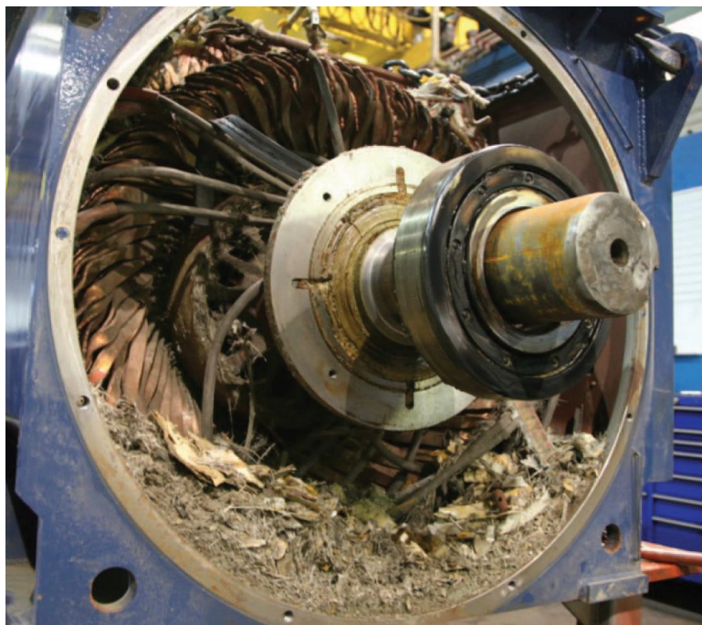
Figure 2.2 Catastrophic failure of a wind turbine generator due to faulty rotor winding [17].
