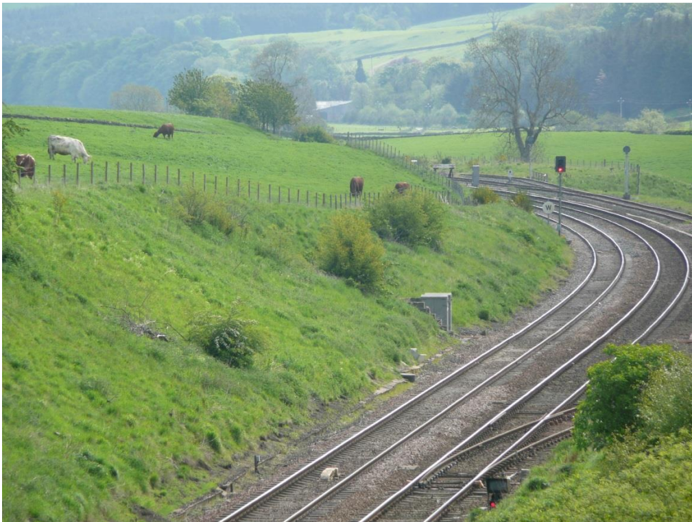
Figure 3.3: South facing earthwork cutting at Whitchester, showing the general undulating terrain. Adjoining fields are used for pasture farming.
