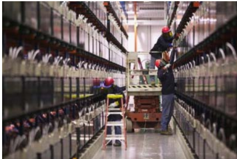
Figure 79 Golden Valley Scheme, Alaska. Capable of supplying 40 MW over 7 min, this scheme is rated the most powerful in the world (photo courtesy of Golden Valley Electric Association)
