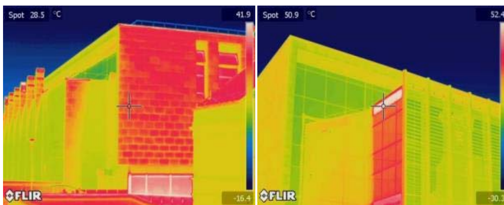
Figure 17 Extreme solar loading in midsummer (4 June 2013-1555 hrs.) showing the great extent of thermal stress that is built up on the external fabric. External air temperature: 16.3^{\circ}\text{C}
