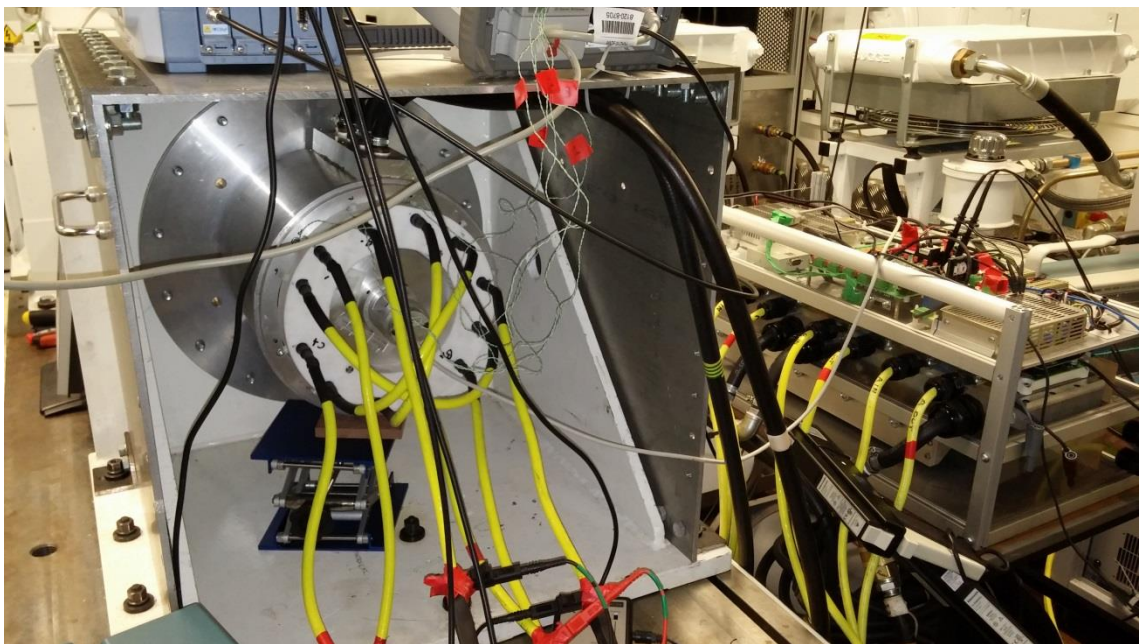
Figure 10-21: Repaired motor on test rig with University developed asymmetric half bridge converter shown in the background.
