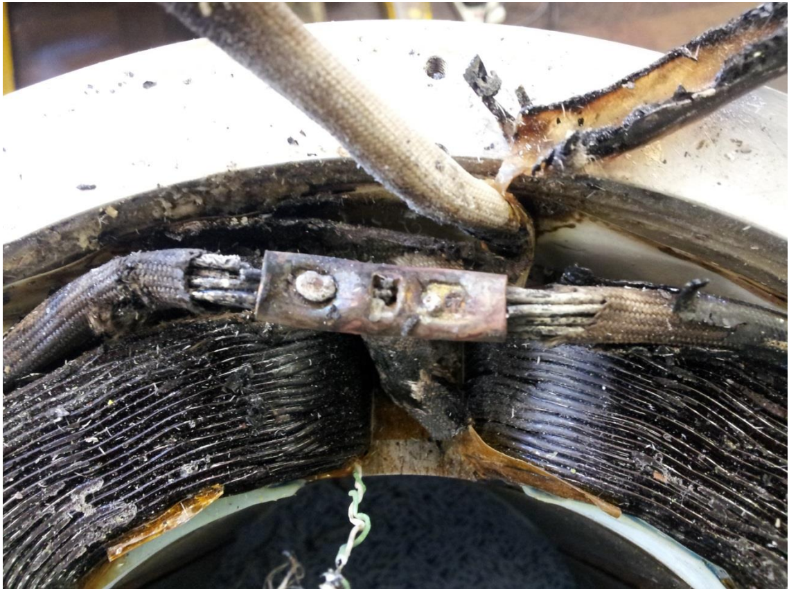
Figure 10-13: Showing damage to the winding interconnections following 5kW winding loss test.
