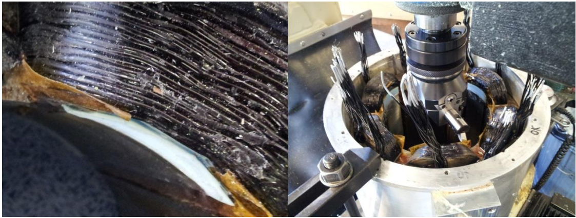
Figure 10-20: (Left) deformed blue-coloured stator end-cap insert and (right) end-cap inserts being machined away as part of motor repair.
