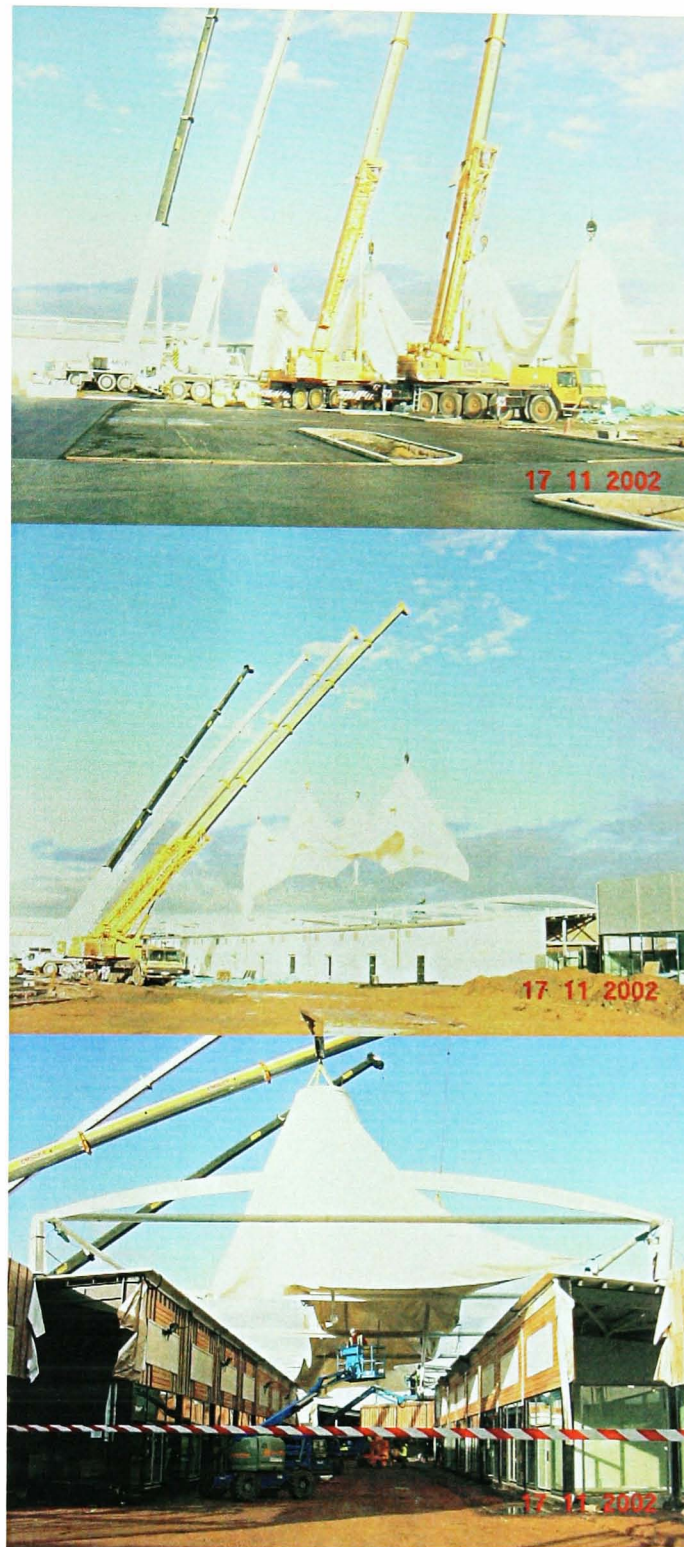
Figure 1-8. Installation of canopy, four linked conics (Dalton Park, County Durham, UK; images – Arup)
