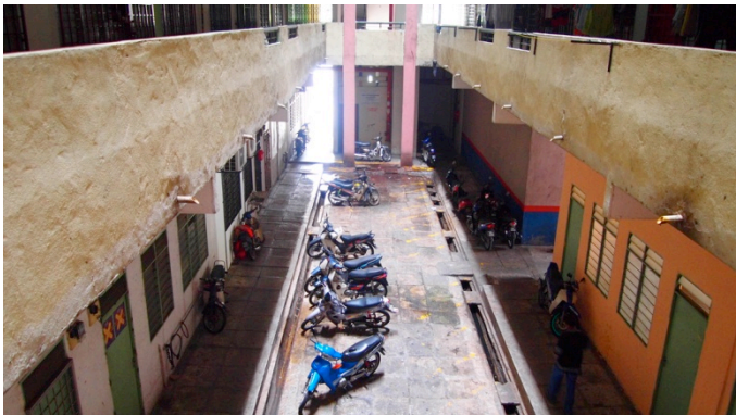
Figure 93 Water from upper levels flow through pipes straight to the ground level instead of being drained out through gutters (Pictures taken by author)
