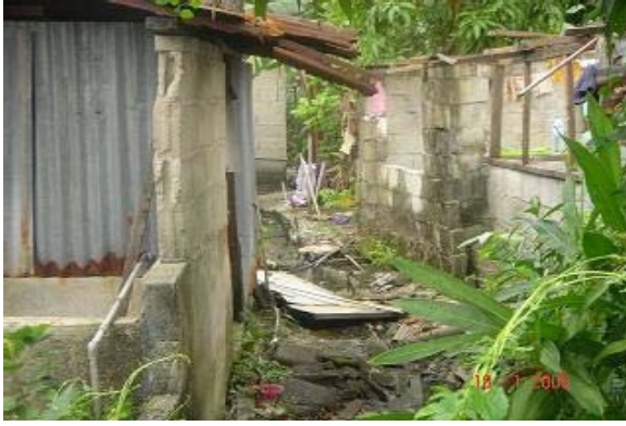
Figure 38 Improper drainage system constructed by the setinggan community (Picture archive from MBPJ)
