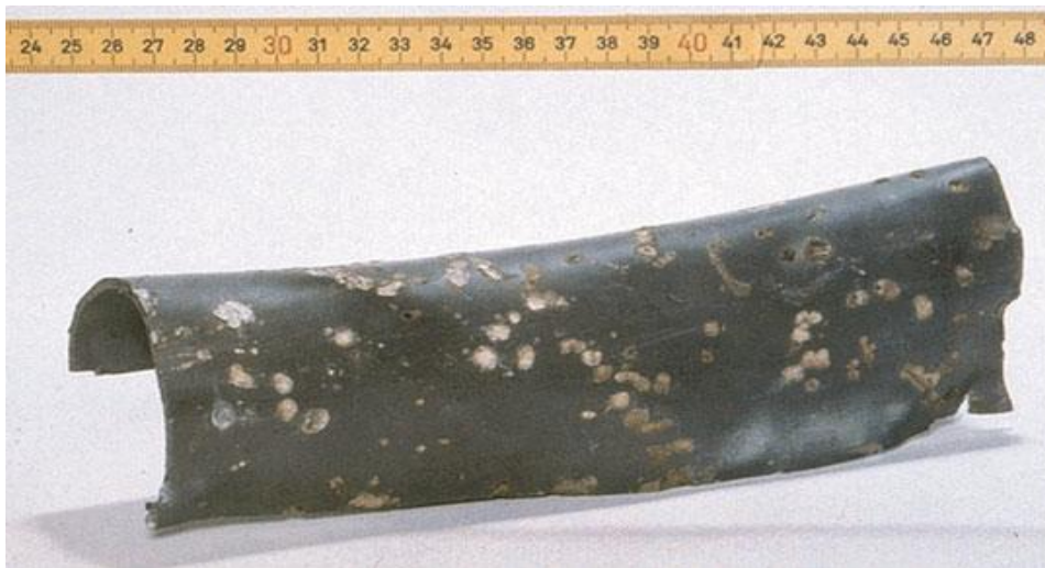
Fig.2.5: Pitting in a lead sheathed cable, caused by stray currents from railways
